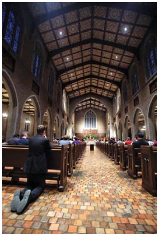
The main chapel features stunning made-in-Detroit Pewabic tiling. The entire chapel underwent extensive cleaning and restoration work in 2009 after a ceiling fire.
