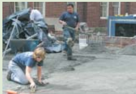
Workers prepare the ground for pavers that will lead the way to a tiled fountain, seen at rear.
